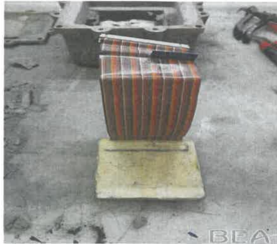
Figure 10: Electrical Flat Ribbon
