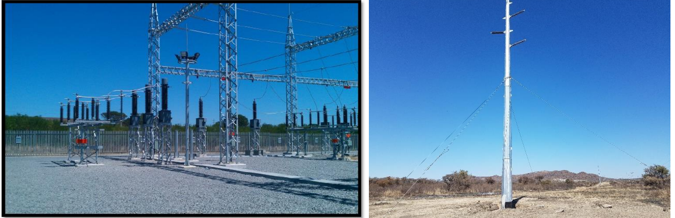
Images of a typical substation Layout and an 88kV Powerline.
