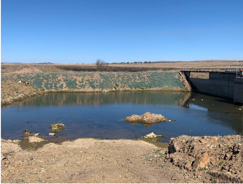
The sewage plant at Ladybrand is derelict and the sewage ends up in the Caledon River, which is the border with Lesotho.
