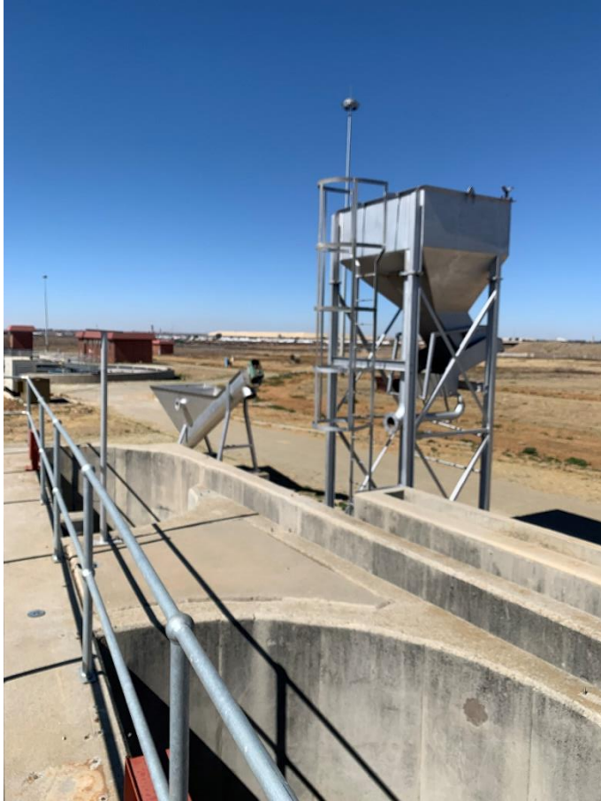
The Thabong sewage treatment plant was built at a cost of R64 million and is currently non-functional with all the sewage flowing into open spaces in the community and eventually polluting the Sand River.
