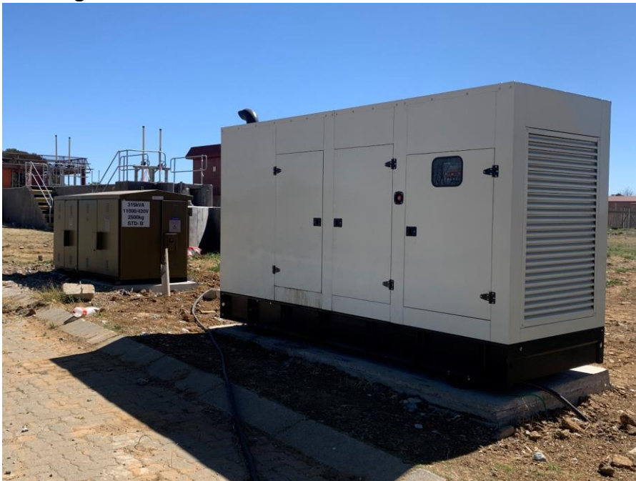
The Thabong sewage treatment plant was built at a cost of R64 million and is currently non-functional with all the sewage flowing into open spaces in the community and eventually polluting the Sand River.
