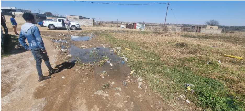
Sewage flows into streets, storm water systems and eventually the Vals River at Bothaville
