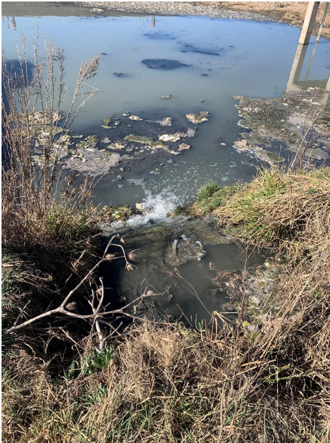
The sewage plant at Ladybrand is derelict and the sewage ends up in the Caledon River, which is the border with Lesotho.
