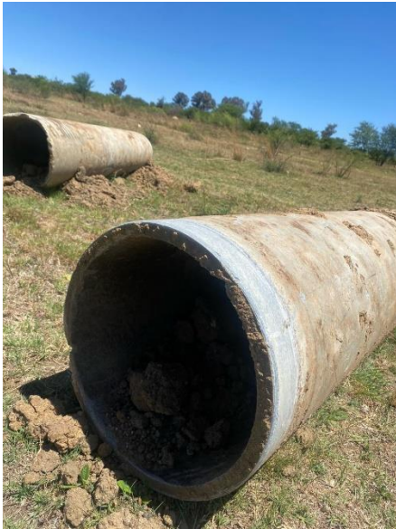
Incomplete water works project to supply water to Parys.
