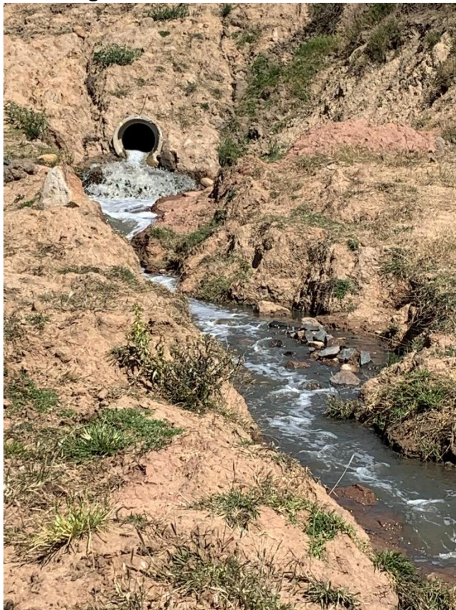
The waste water treatment plant that serves Mashaeng at Fouriesburg is dysfunctional with raw sewage flowing through streams into the Little Caledon and eventually the Caledon River.
