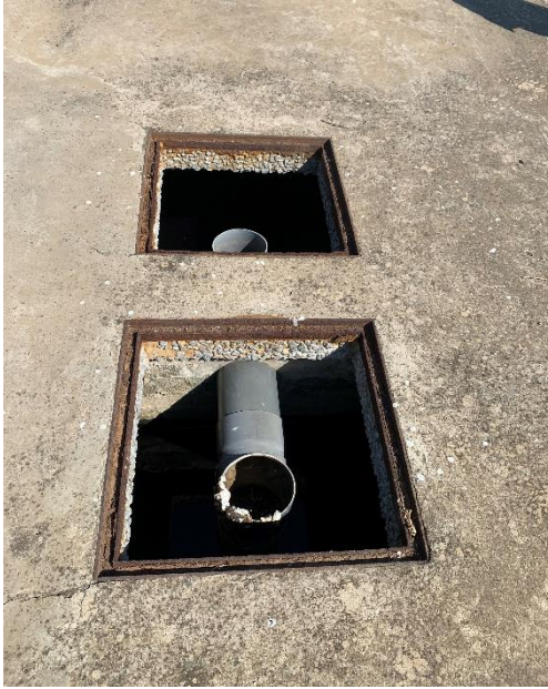
The waste water treatment plant in Ntha at Lindley was built and remains dysfunctional.
