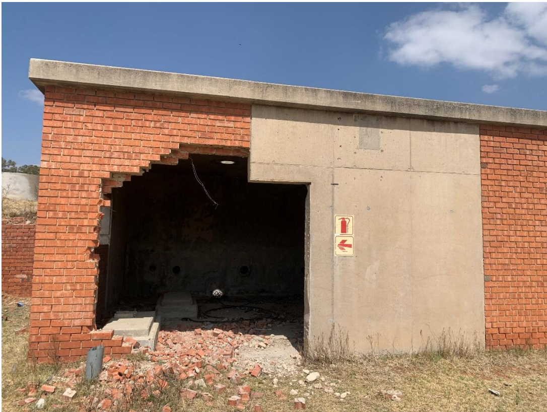
The Odendaalsrus sewage treatment plant was refurbished in 2010 to the value of R16 million. Today it is derelict and vandalised with all the sewage flowing into the Sand River and is budgeted to cost R185 million to rebuild.
