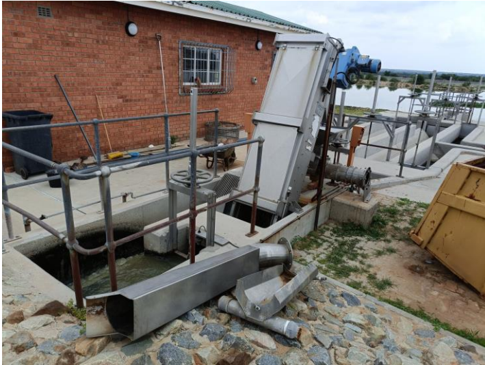
Broken equipment at the sewage plant
