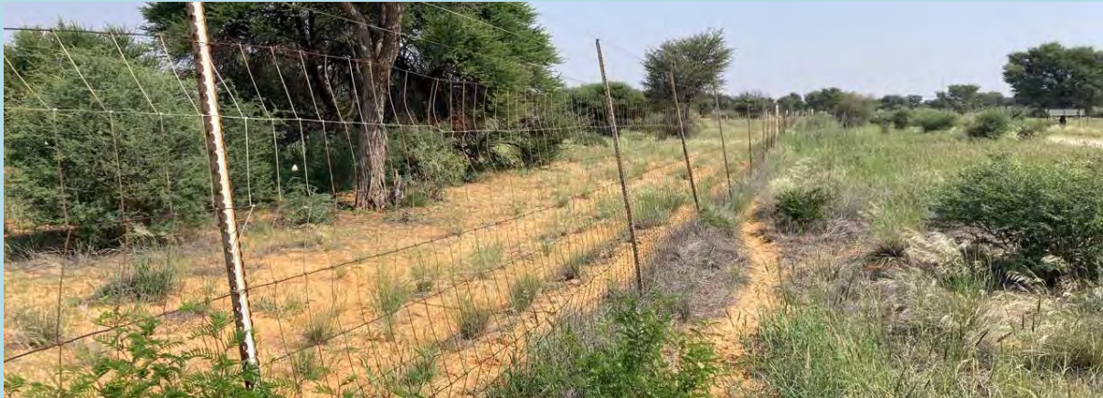
Molopo's fence in disrepair
